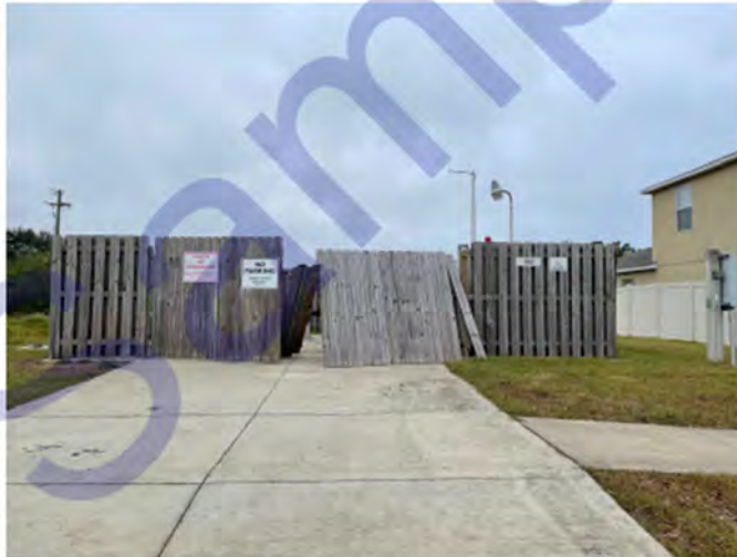
Broken Gate at Lift station
